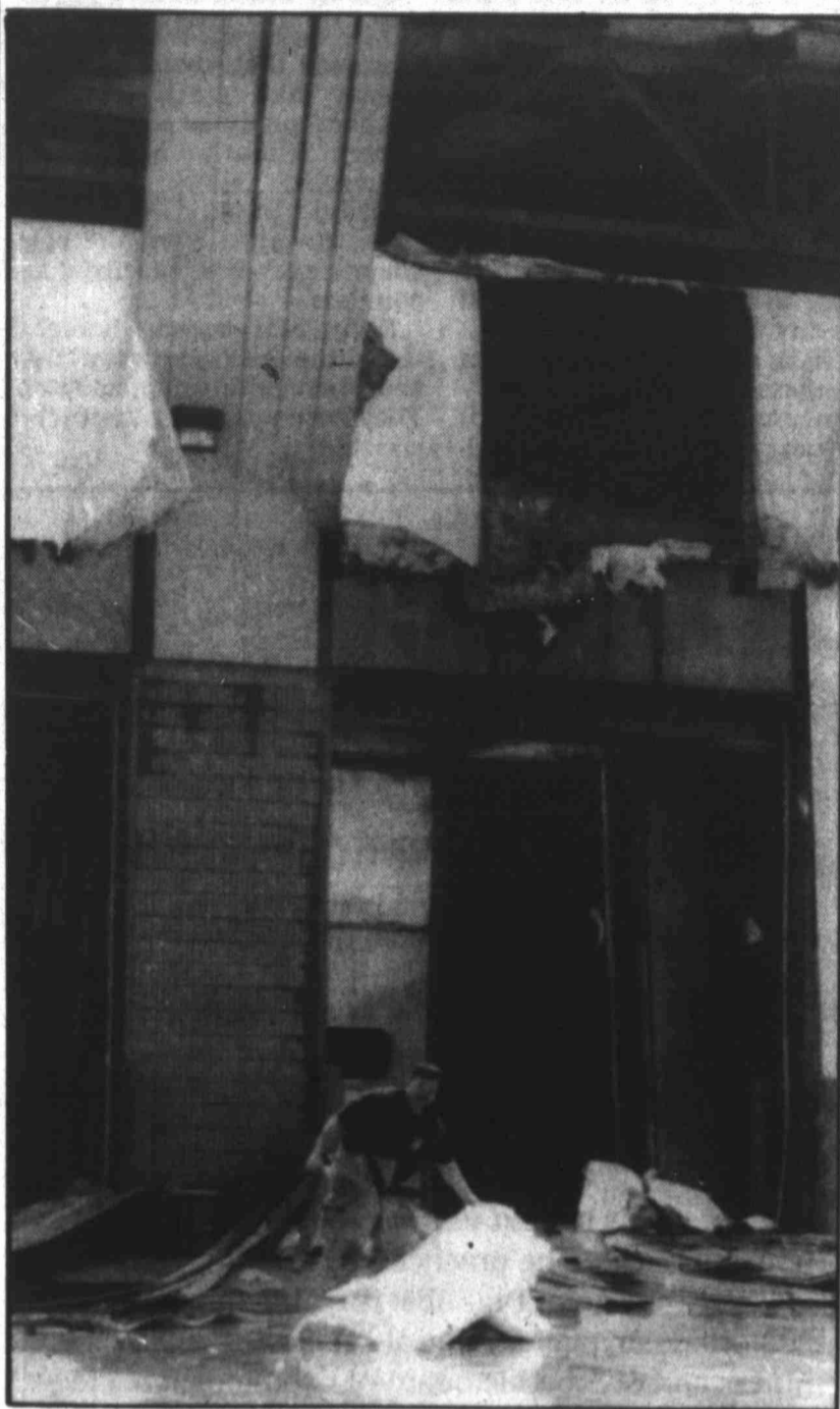
A Fort Bragg firefighter moves a piece of insulation to roll up a hose after an explosion in a paint booth blew siding and insulation from the sides of an Installation Material Maintenance Division building on Fort Bragg, N.C. Wednesday. The blast injured 22, severely burning two workers.
