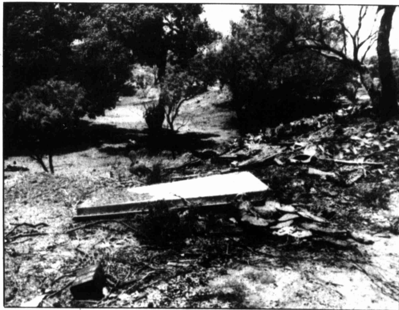
The cleanup of the canyon along Pennsylvania and Lancaster streets, north and west of the First Church of the Nazarene, has created a controversy after neighbors complained. Church officials have asked that the work be done. Residents attended the Big Spring City Council meeting to discuss the issue, both pro and con.
