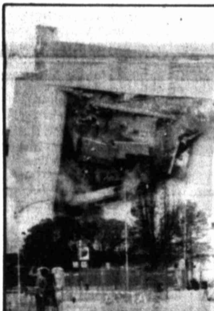
The Alfred P. Murrah Federal Building falls in a cloud of dust as it was demolished by explosives Tuesday.
