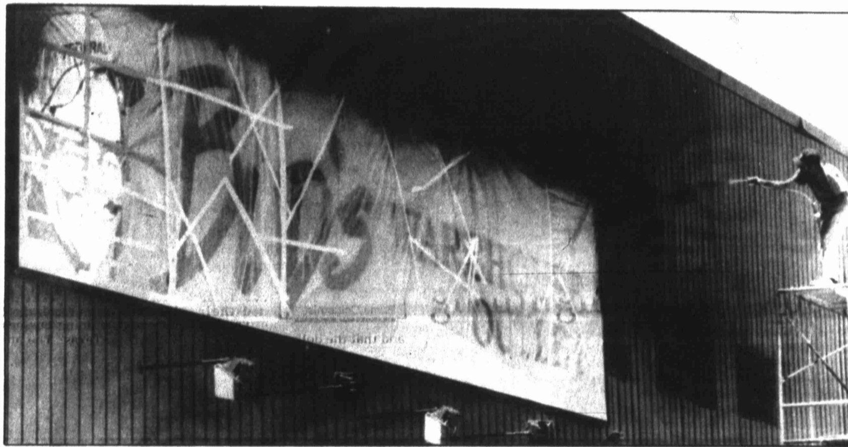
John Cruse sprays red paint onto the old Wal-Mart building Tuesday afternoon as work continues on the conversion to the Bud's Warehouse Outlet. The store is expected to open Wednesday, May 3.
