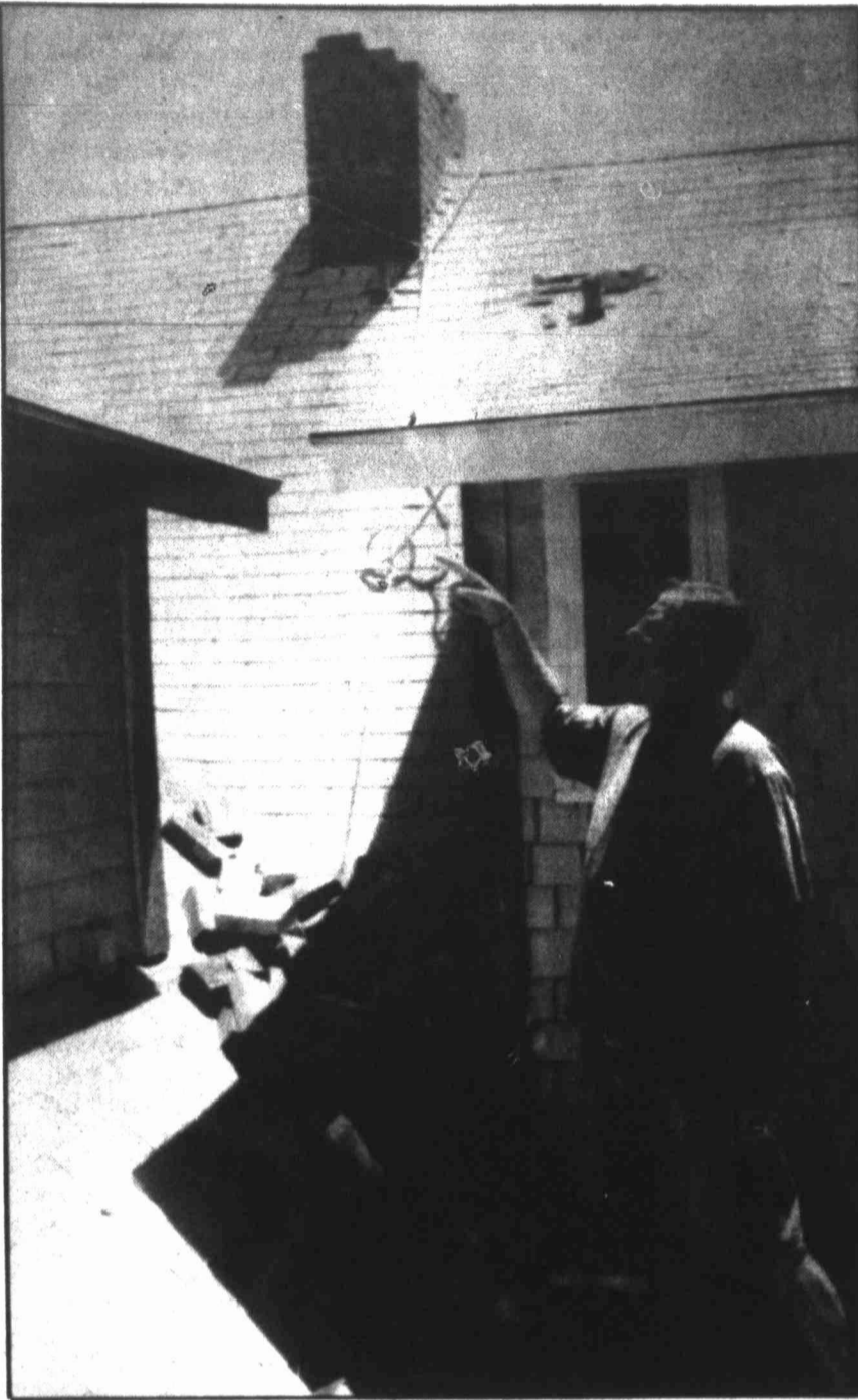
Bob Hext surveys the damage to the chimney on his house in Alpine Friday after an earthquake with a magnitude of 5.6 hit Thursday. The quake, centered about 20 miles outside of Alpine, caused two minor injuries, some structural damage and triggered a few fires.
