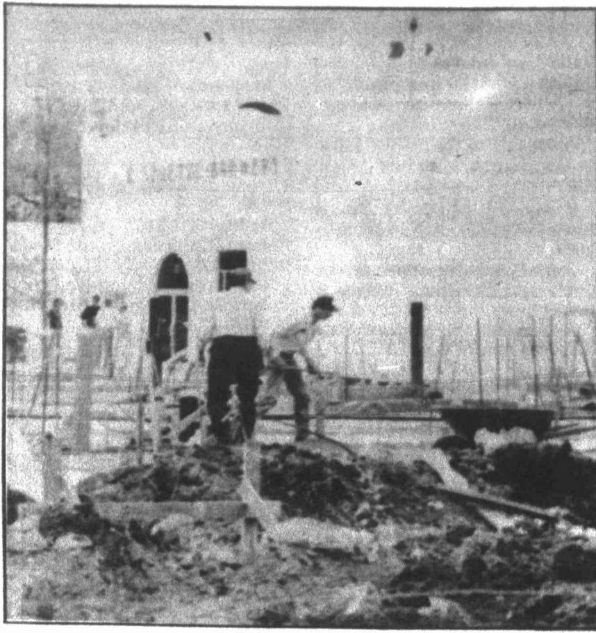
Associated Press photo Workers set the foundation for a new brew house at the Spoetzl Brewery in Shiner. The addition will double the brewery's production of its three types of beers.
