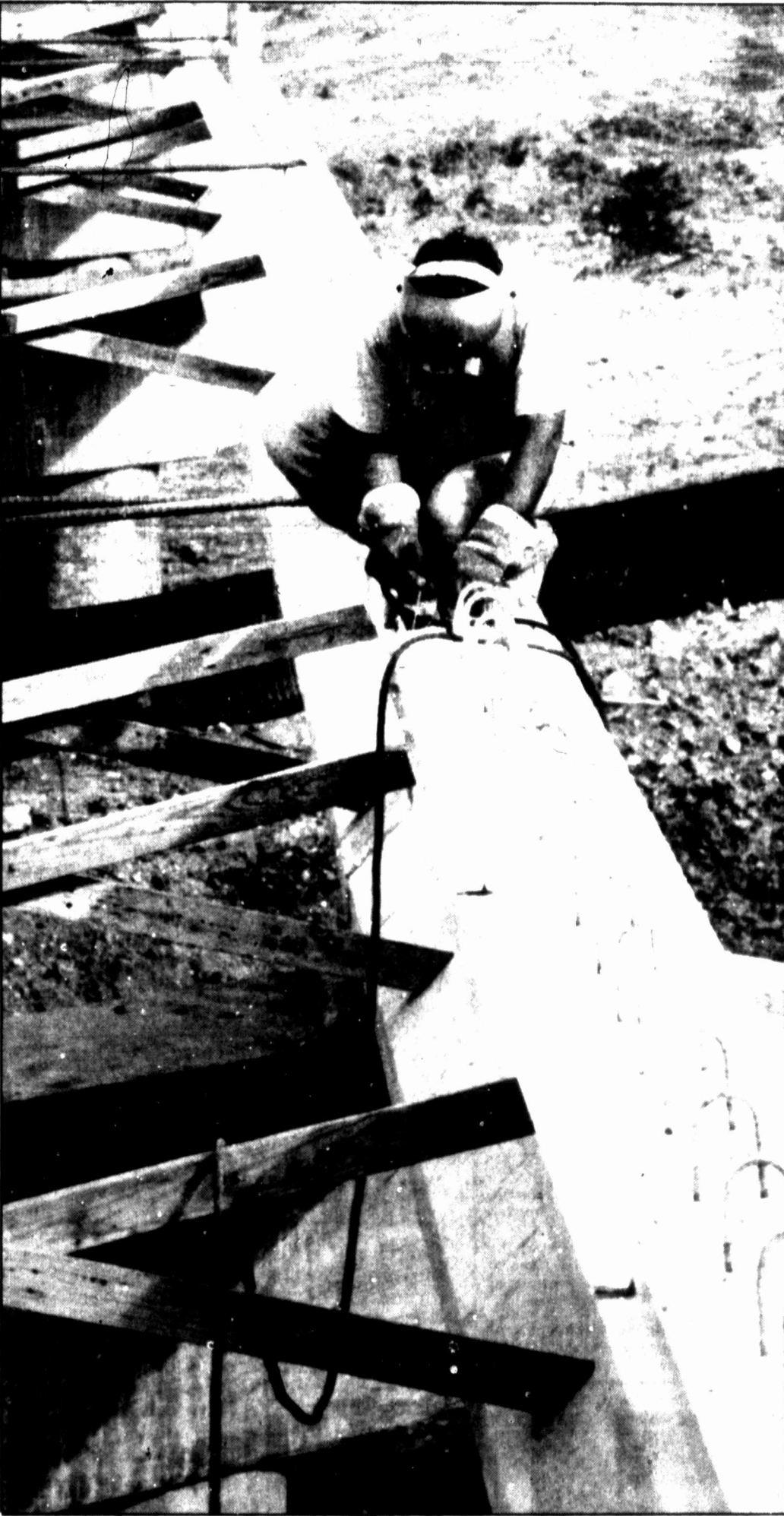
A worker crouches down on a concrete beam high above the ground to weld a wire into place as work continues on the Interstate 20 bridge widening project Tuesday afternoon.
