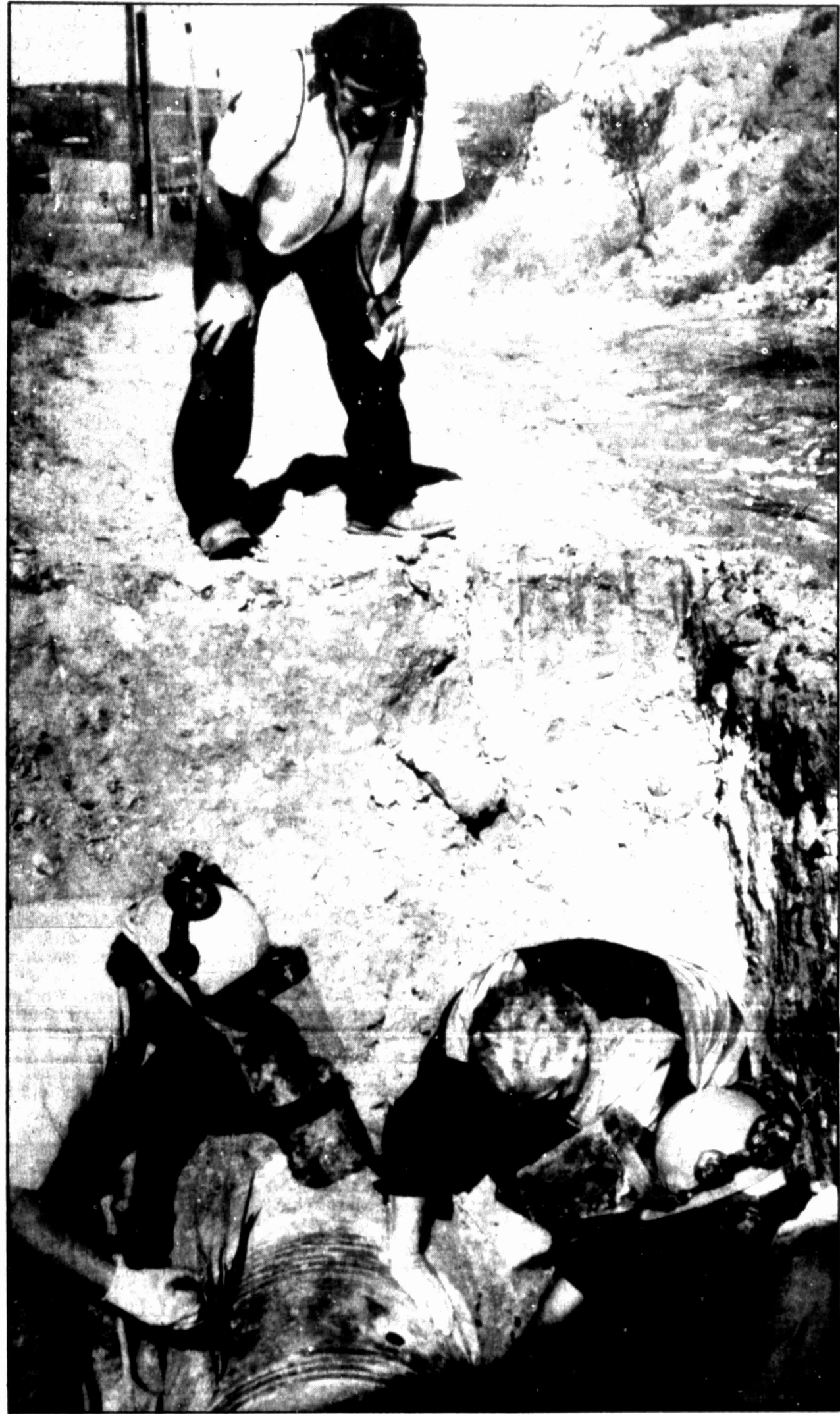
City of Big Spring Public Works Director Tom Decell and other workers look at a hole in a 20-inch water main Saturday morning. The hole, caused by exterior corrosion and leaking 10 gallons of water per minute, forced the city crews to shut down much of the water supply on the east end of Big Spring, including Big Spring Mall.
