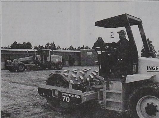
GRADING WAS begun this week at Parmer County Community Hospital in preparation for the construction and remodeling of the facility. At left is Tony Mureuia of Wiley Construction of Amarillo,
