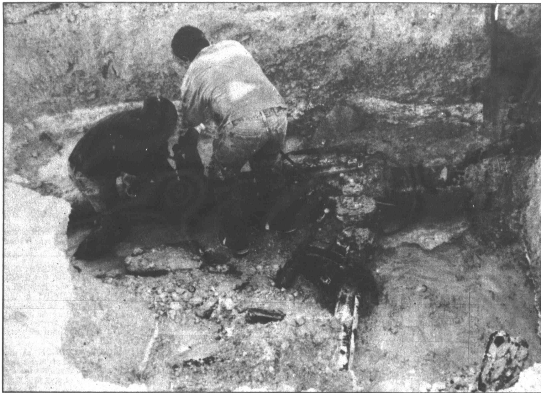
City crewmen work to fix a waterline leak at 15th and Princeton that left a good portion of Big Spring without service for several hours this past weekend. The city will receive an update from Pitometer & Associates this week about that city's water loss problems.
