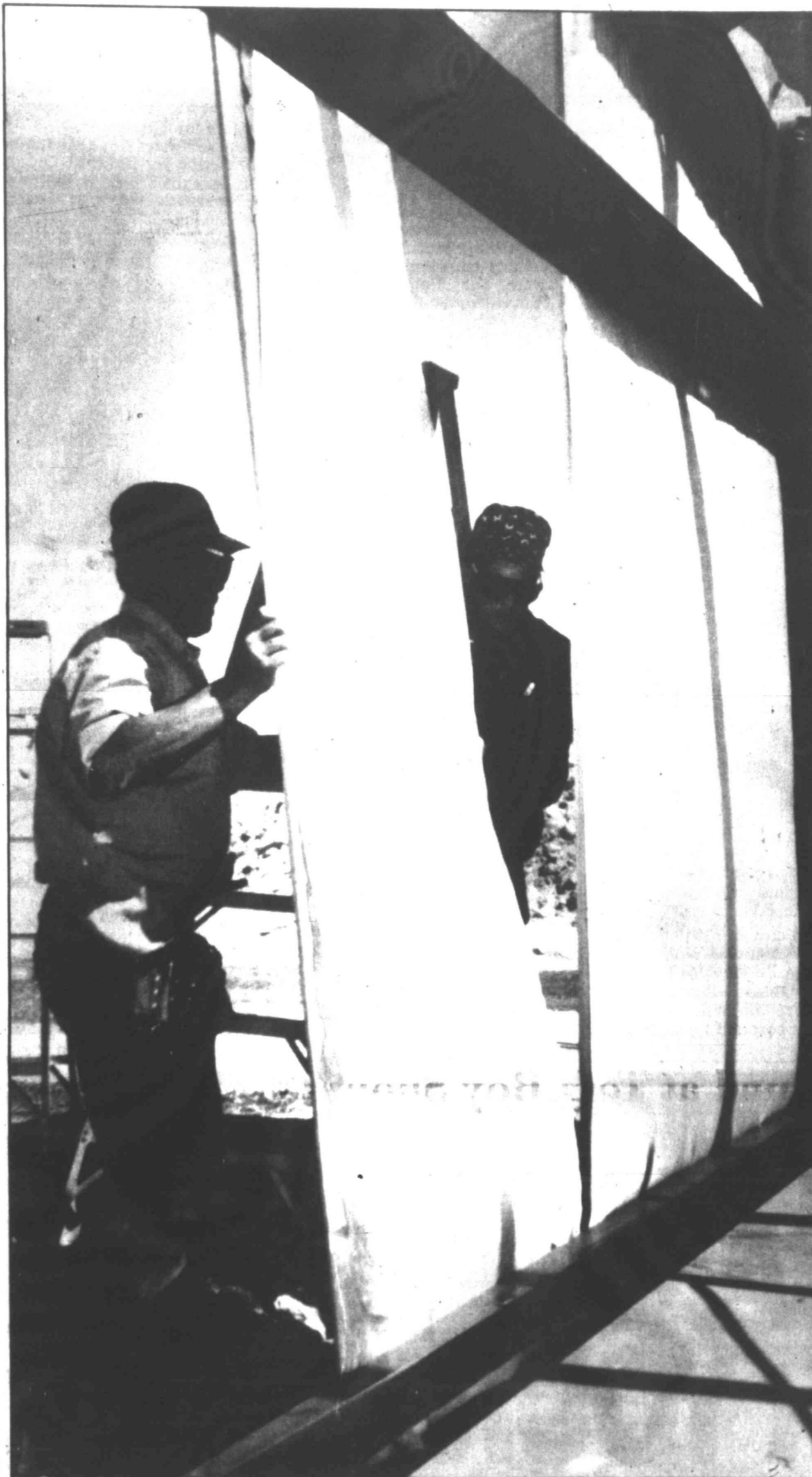
Jack Tibbets and Carl Condray put up a piece of the exterior wall of the new City of Big Spring landfill office Thursday afternoon. The building will have a weigh station to weigh the amount of refuse that is being brought into the facility.
