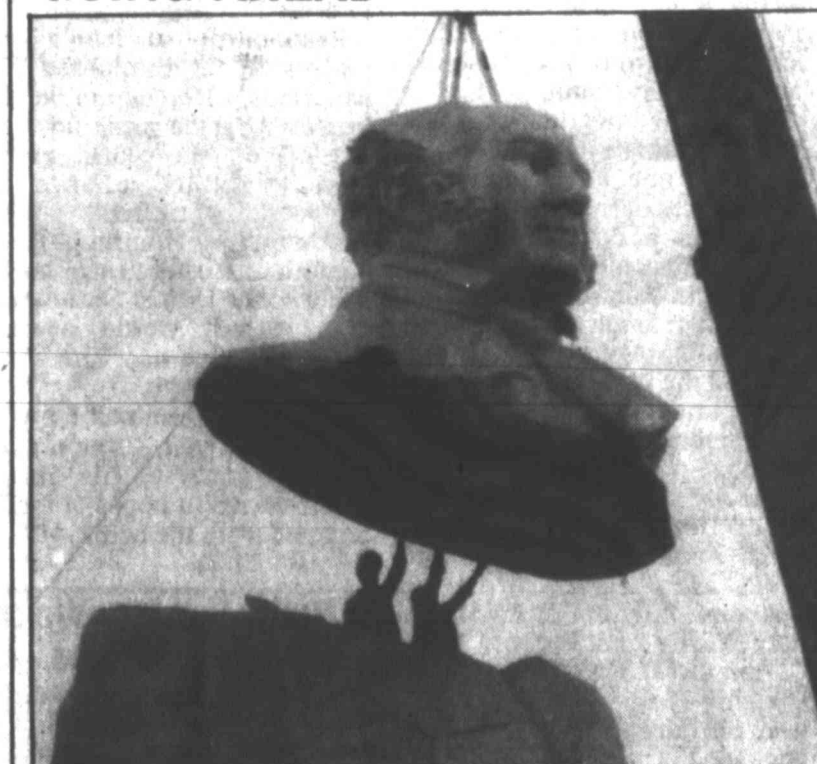
Workers guide the head section of 67-foot tall concrete sculpture Sam Houston to the correct position recently in Huntsville. Houston was the first president of the Republic of Texas. The statute, designed by David Attickes and donated to the city of Huntsville, will be dedicated Oct. 22.
