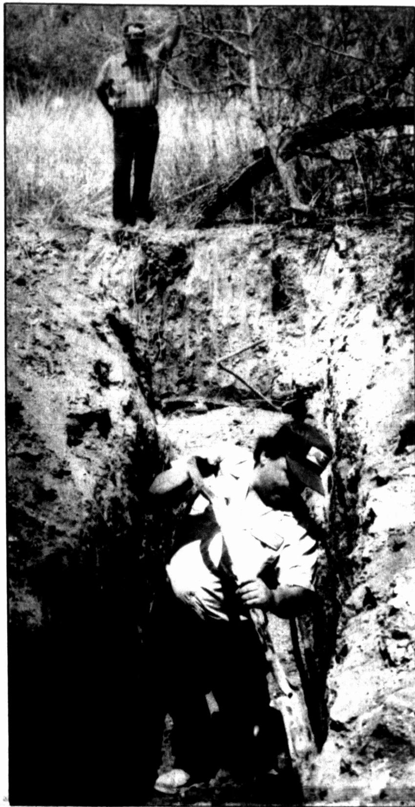
Property owner Bill Stone looks on as City of Big Spring worker Gary Walter digs out a water pipe in a trench on Cole Street Wednesday. The abandoned pipe had been spewing water into Big Spring Creek for over four years.
