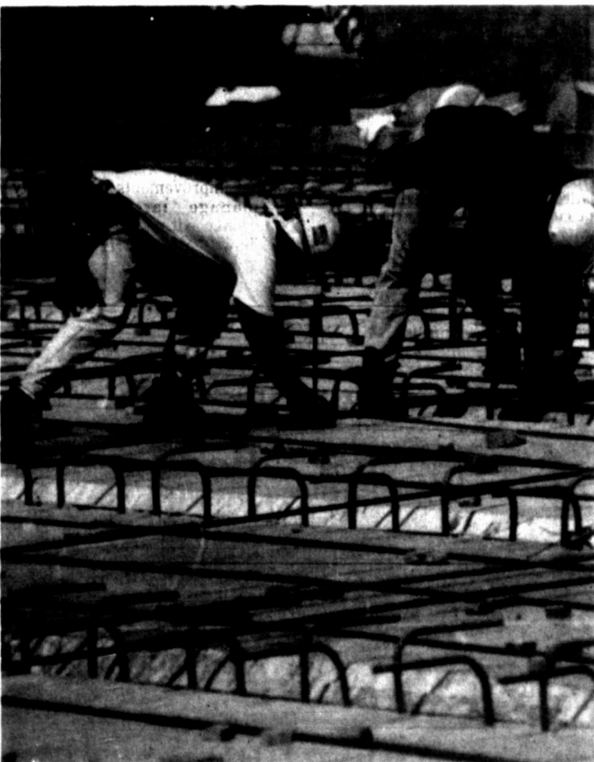
Workers put steel frame work into place before the pouring of concrete on the new bridge of the Santa Monica Freeway in Los Angeles. Workers put in 12-hour shifts, seven days a week, during the rush to rebuild the freeway since the Jan. 17 Northridge earthquake.
