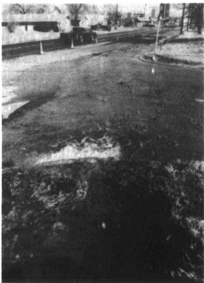
City crews work to fix a water main break which Assistant City Manager Tom Decell describes as a "timebomb," which is very costly to the city in terms of equipment, manhours and maintenance.
