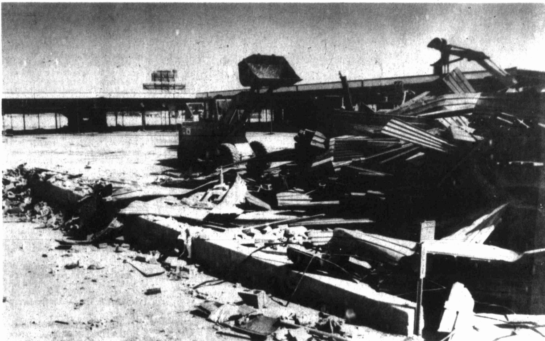
There is not much left of Highland Mall except for the rubble to be hauled off. Highland Mall was selected as the site of the new Wal-Mart
