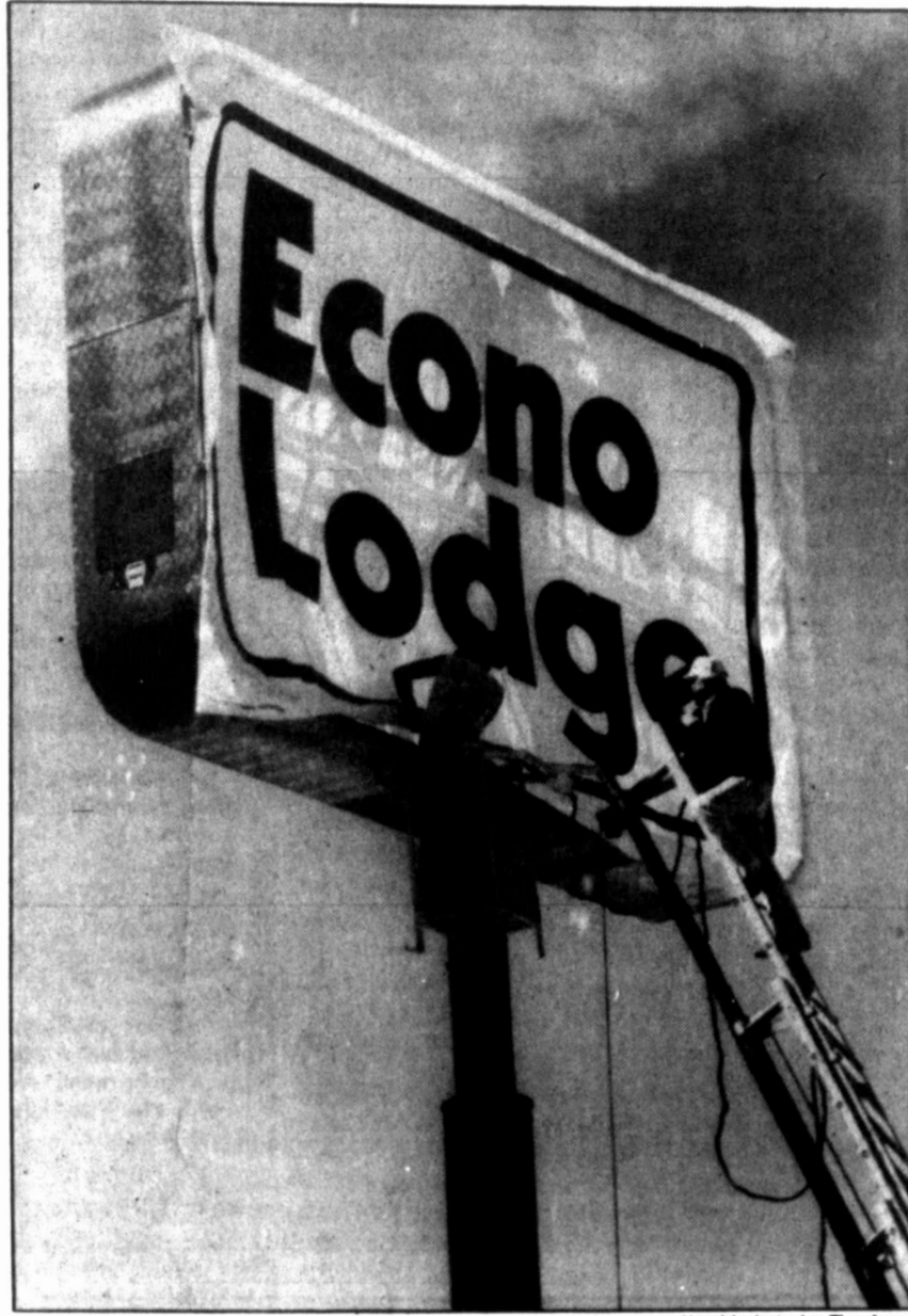
Flo-Lite Sign Company employees work on installing the Econo Lodge sign along the north service road of Interstate 20 Tuesday afternoon. The motel is slated to have a ribbon-cutting ceremony Wednesday, and the sign is of a trampoline material to withstand the strong West Texas winds.
