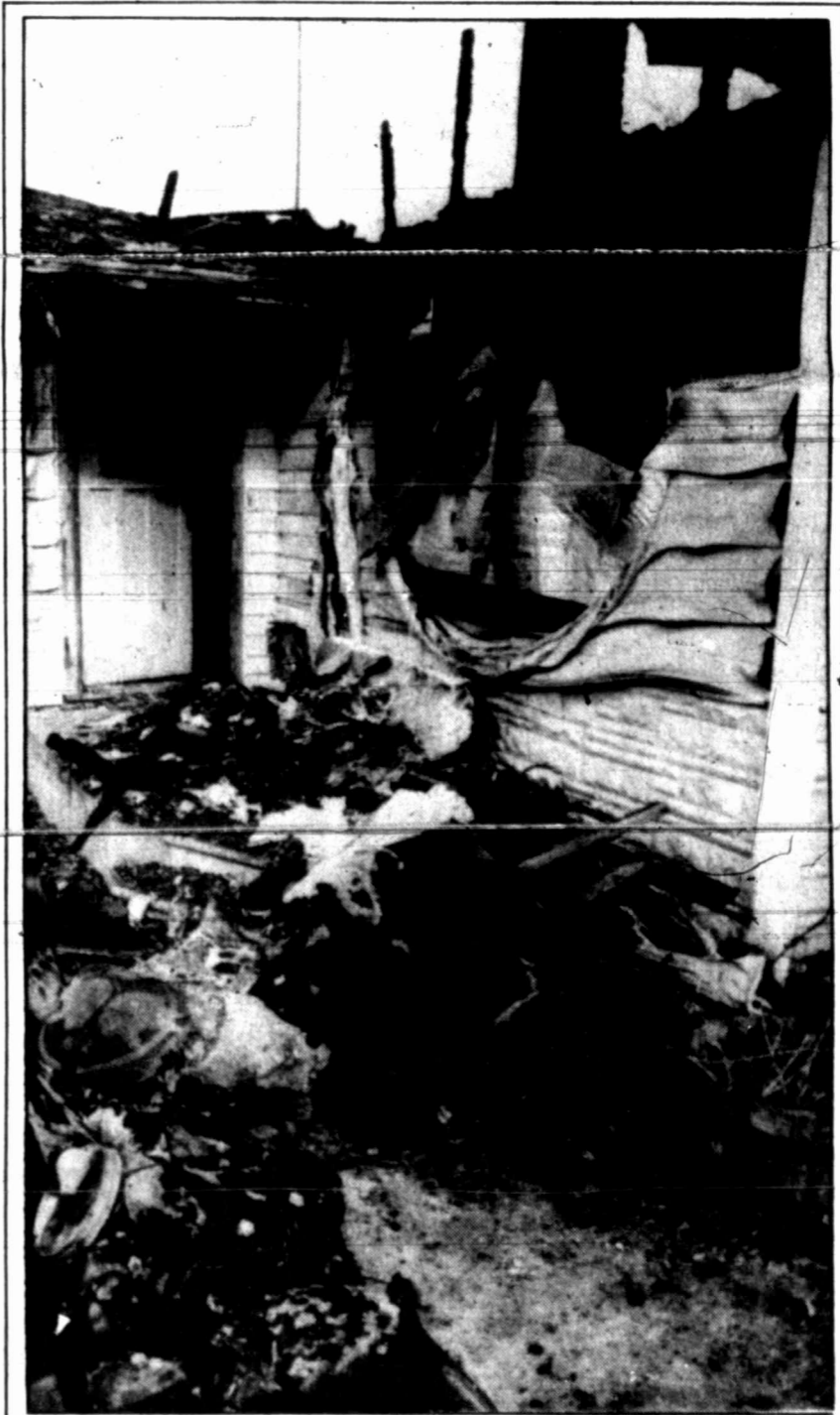
A burned couch and a partially-melted Christmas tree sit near the front door of a home in Forsan that was gutted by fire during the Christmas weekend.
