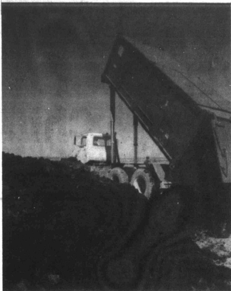
A truck dumps a load of sludge onto Sierra Blanca, ranchland earlier this month after arriving from New York by rail.
