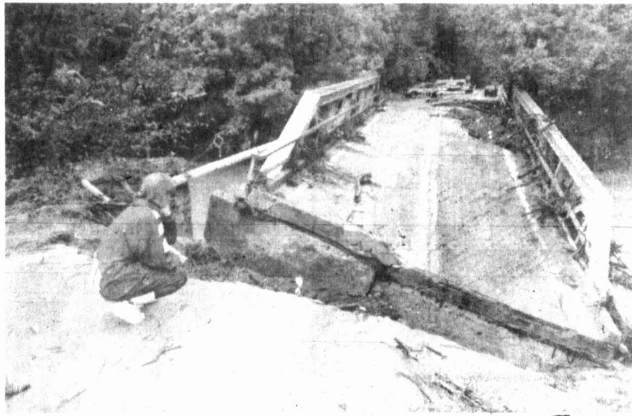
Tracey Vortman looks over the destruction of the bridge over KeKrs Mill Road in St. Louis County, Mo., Thursday. The bridge collapsed Wednesday night after being covered by flash flooding in the area.
