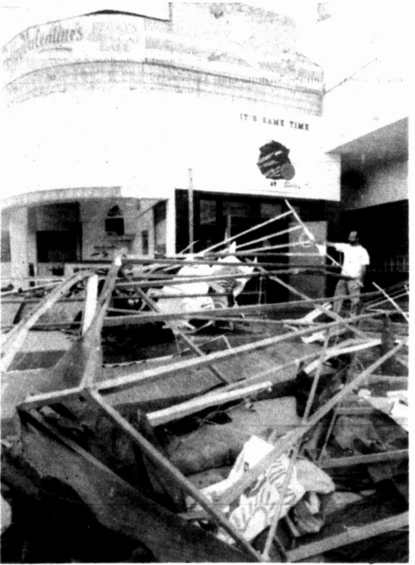
Kirk Lewis, manager of Bobby Valentine's Sports Gallery Cafe, looks over the damage sustained after high winds blew through north Arlington Monday morning. One person in a nearby hotel was injured in the early morning storm.
