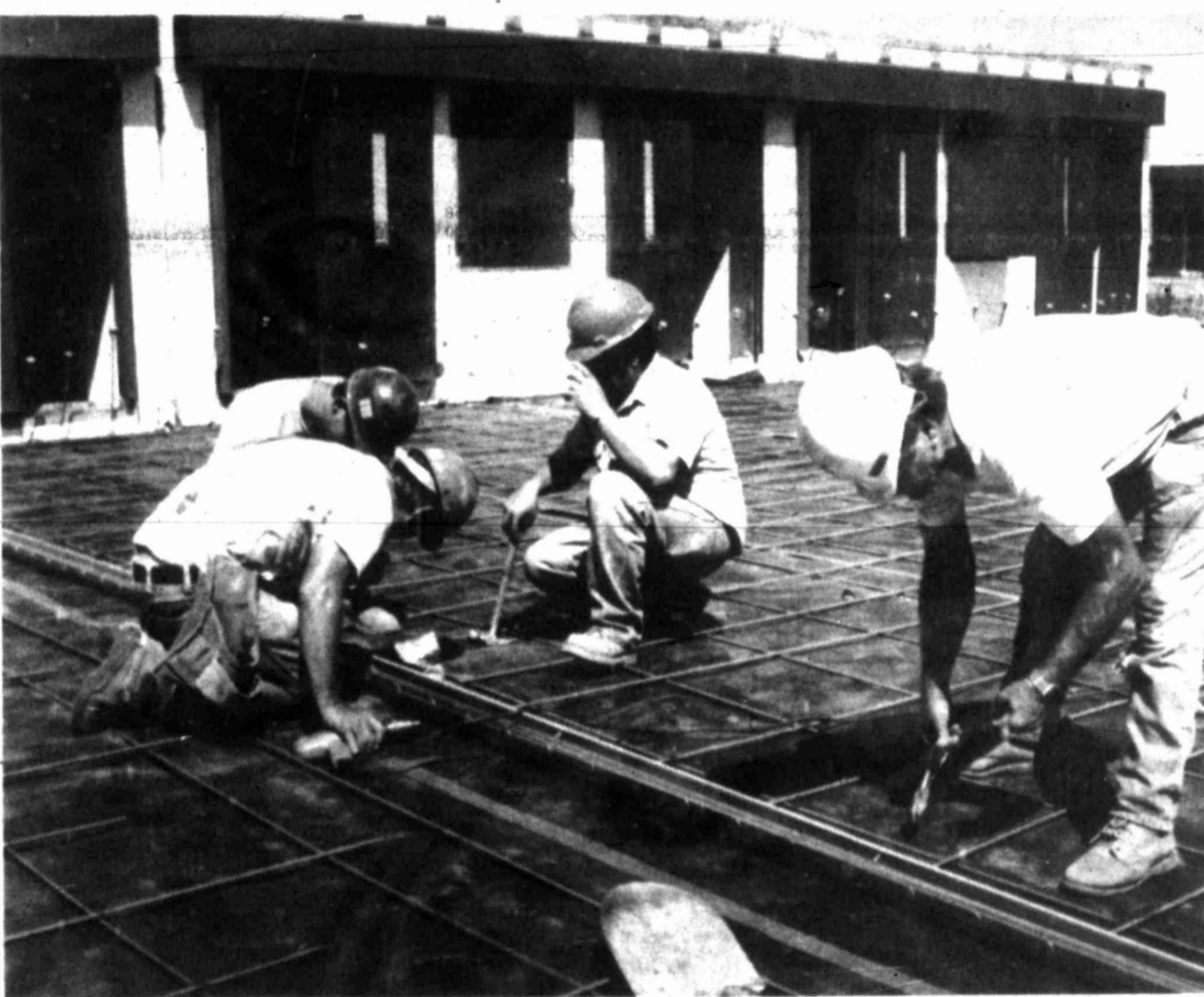
The D.W. "80" John Wallace Unit construction is 16 percent completed. Twenty-seven cell modules are erected as well as 80 percent of the perimeter fence. Concrete patrol roads are 90 percent completed with underground utilities about 80 percent. First metal building structures arrived Monday. Completion date is May 1994.
