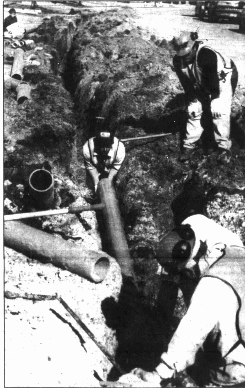
City of Big Spring workers lay water lines in the Capehart area Tuesday afternoon as part of the pipe replacement project currently underway. Work has reportedly been slowed by thicker-than-expected concrete driveways.
