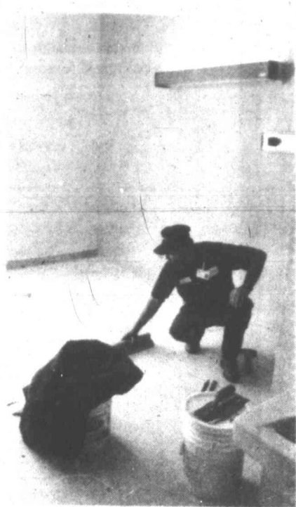
Scenic Mountain Medical Center employee Steve Larkey cleans the floor inside a newly-renovated third floor room at the hospital Monday afternoon. Floor tiles now replace stained carpeting inside the rooms.
