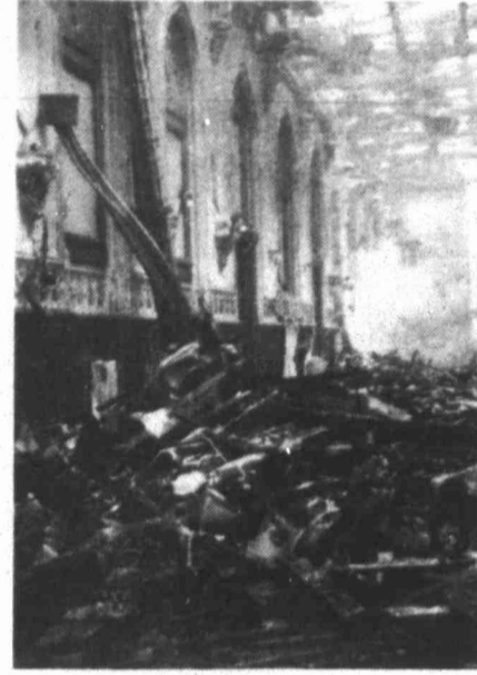
The damaged interior of St. George's Hall, inside Windsor Castle, is seen Saturday following a fire which started Friday and caused millions of pounds worth of damage to the 900-year-old castle.
