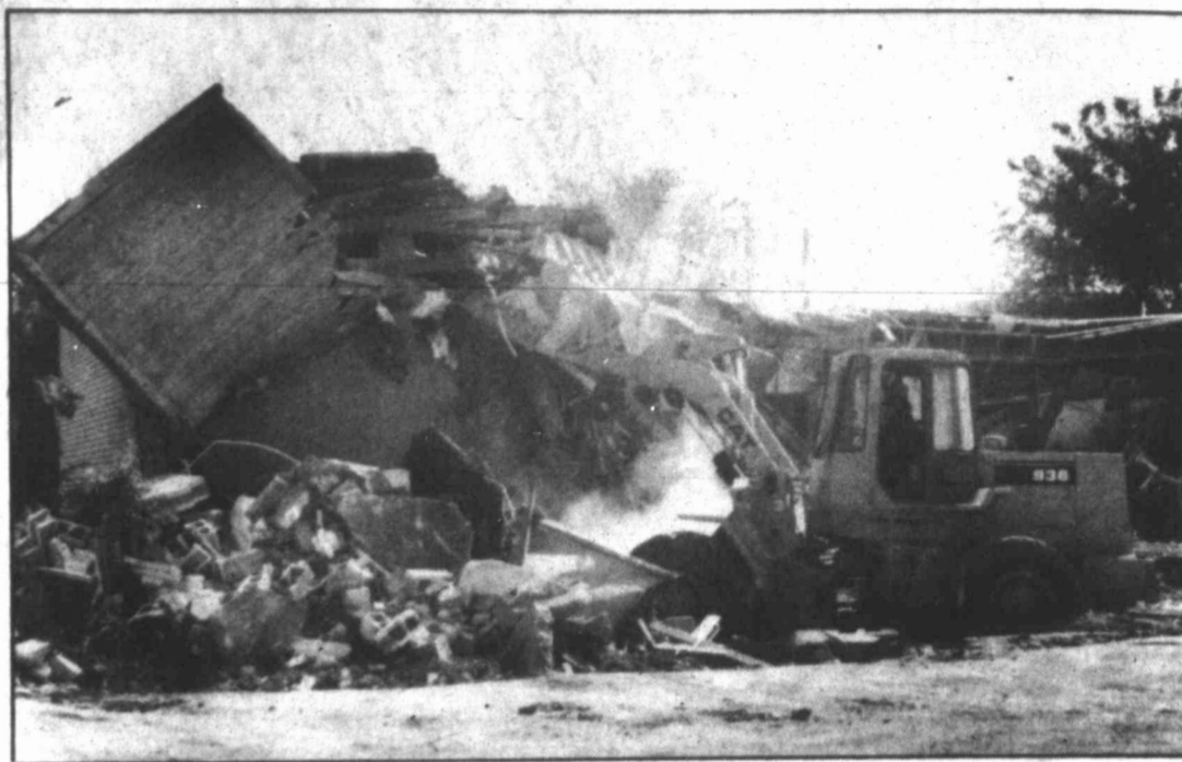
Bulldozers work on the demolition of the old Cowper Clinic building Monday. The building, about 50 years old, is owned by St. Mary's Episcopal Church.
