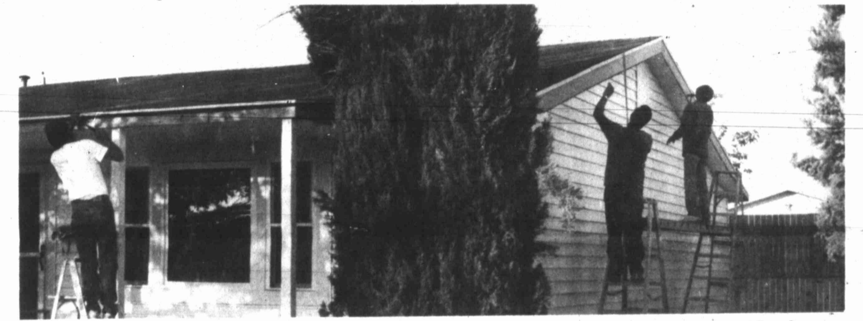
The professionals of Four Seasons Insulation and Siding, Inc. installs wall siding, soft fascia overhangs on a area home. If you're interested in complimenting your home with beautiful new siding, vinyl or steel. Call the professionals at Four Seasons Insulation and Siding, Inc. at 264-8610.
