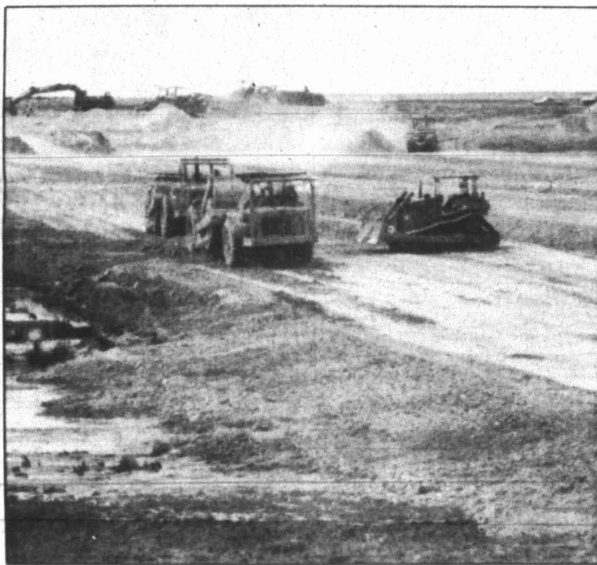
Heavy equipment rumbles over a recently-erected earthen dam along Sulphur Springs Draw this week. The dam will rise an additional 25 feet before completion in October.
