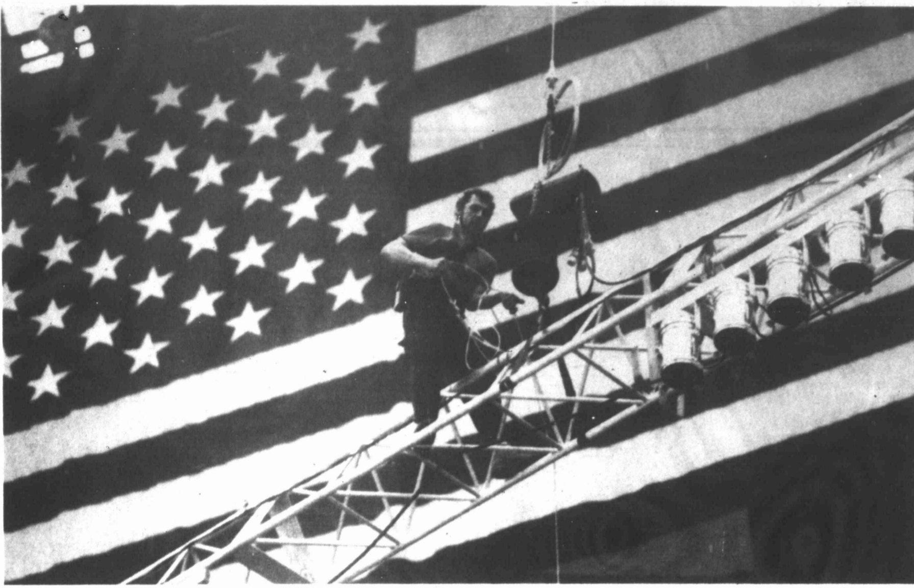
Michael Miller, a rigger at the Republican National Convention, hangs from a lighting truss in the Houston Astrodome where the convention will begin Aug. 17. There will be 2,100 lighting instruments in the dome when the job is completed.
