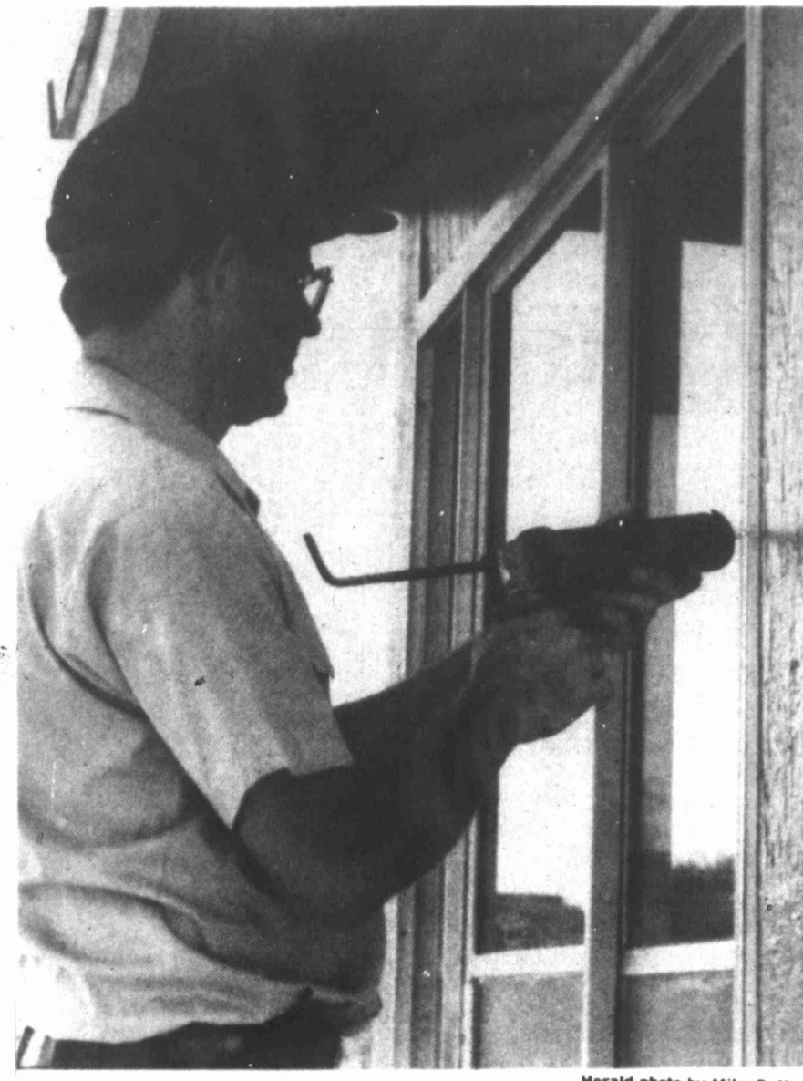
Big Spring State Recreational Area park manager Michael Young works on the park's new entrance booth. Young says the booth, along with a new fee drop box, will improve both park security and the park's ability to collect visitor fees.
