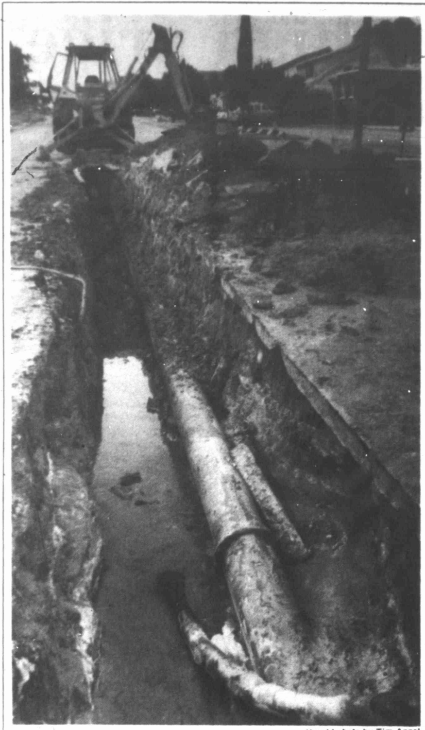
Fixing the leak A 12-inch water line break at the intersection of 7th and Johnson streets left area residents without water this morning. The corroded cast iron bell joint gave way at approximately 2:14 a.m. this morning and approximately 30-40 feet of pipe will be replaced.
