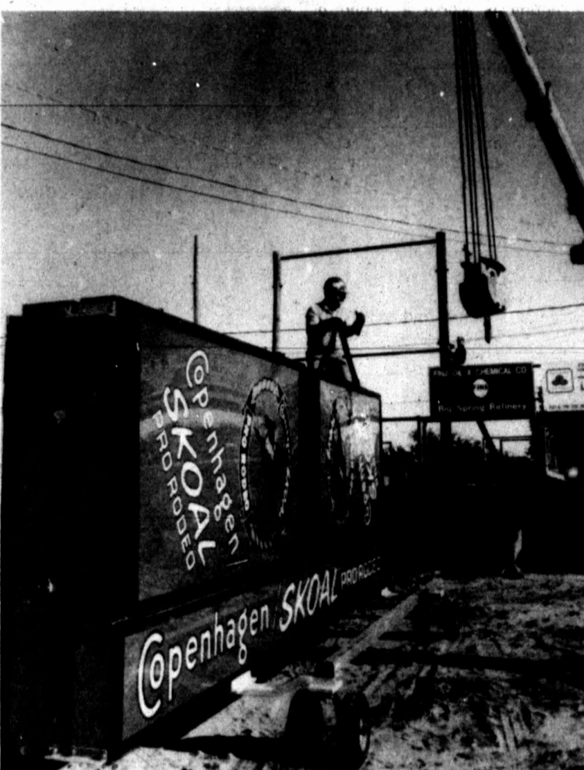
Cathey Construction worker Pat Lamb sits atop the Copenhagen/Skoal rodeo scoreboard and motions the crane operator to swing the boom closer to him as workers prepare the Rodeo Bowl for the 59th annual Big Spring Rodeo beginning Wednesday. The scoreboard, complete with graphic capabilities, will be the first used at the rodeo in nine years.
