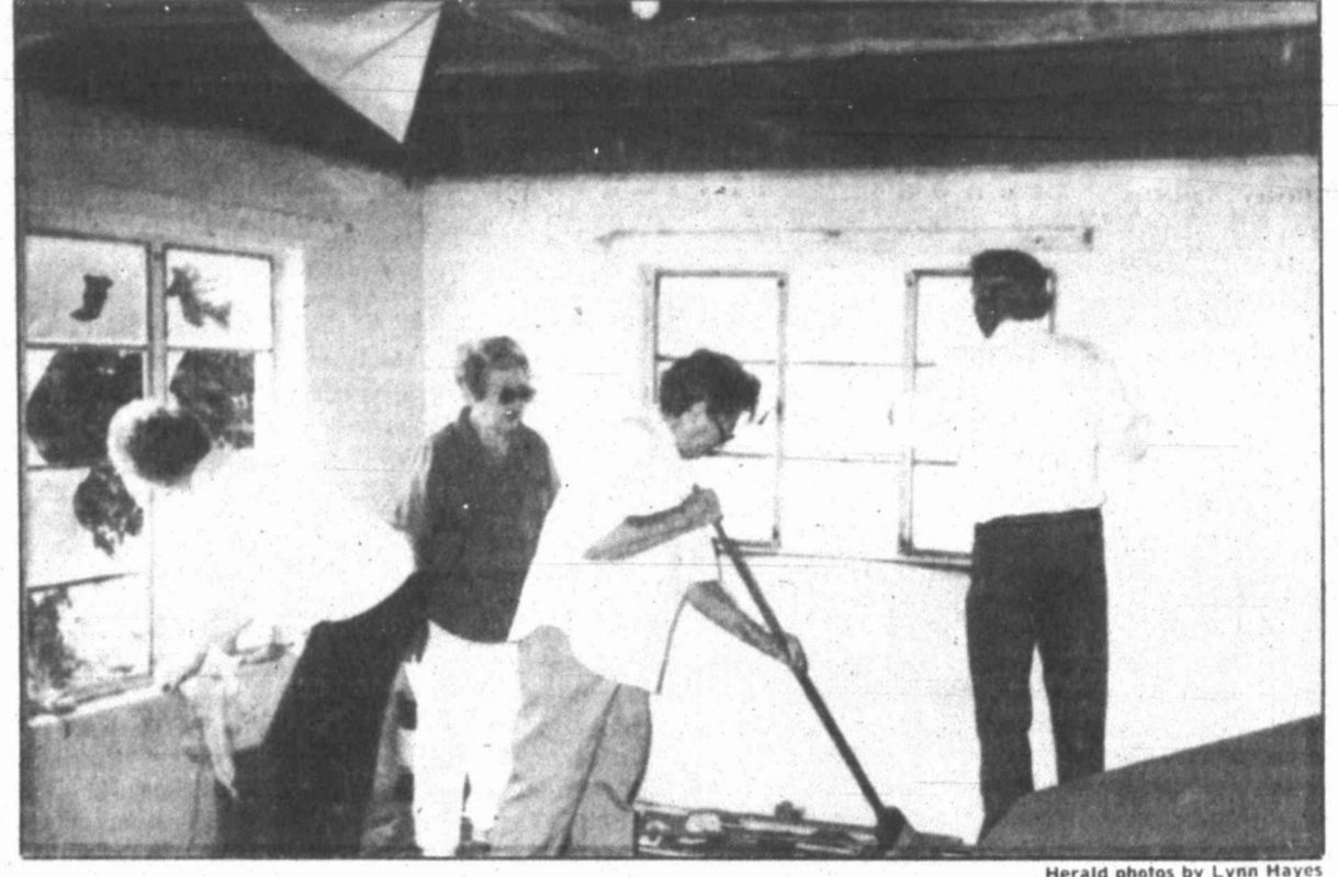
Mona Lou Tonn, Claudene Baker, Trudy Carter and the Rev. Arnold Tonn begin repairs on the building that will be used as a gathering place for the hungry.
