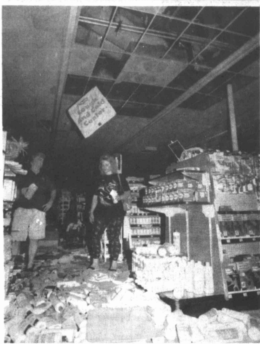
At Cravan, left, and Mary Merrick, managers of a drug store in Desert Hot Springs, Calif., look over damage to their store caused by an earthquake Wednesday night. The quake, which measured 6.1 on the Richter scale, was centered in desert communities 100 miles east of Los Angeles. No deaths or major structural damage has been reported.
