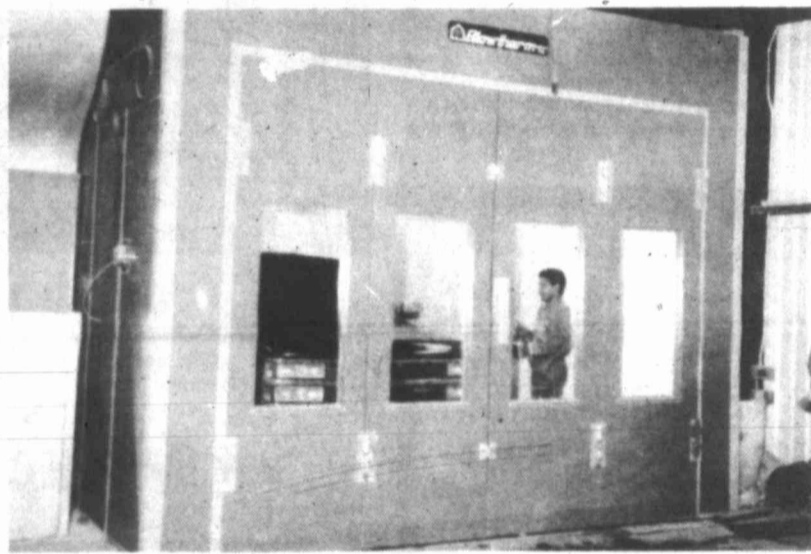
Pictured above: Leo Gonzales (painter) working on customer order in one of two Blowtherm Ultra downdraft paint booths. Call Pat Gray's for more information today. 263-0582.
