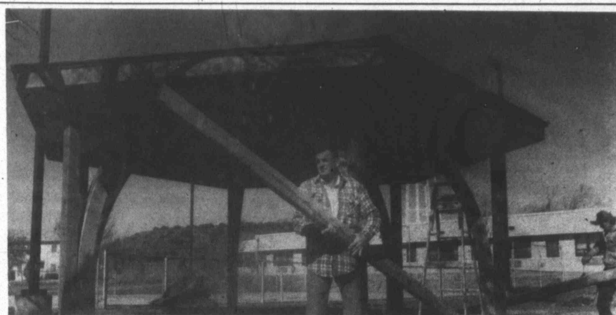
In 1991, Big Spring V.A. Medical Center's pavilion was constructed to provide a covered shelter for veterans, visitors, volunteers and employees to enjoy meals and breaks. The con-
