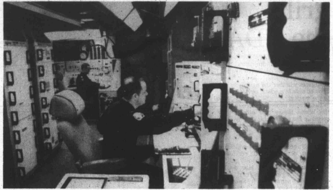
Capt. Jeff Schaff, left, and 2nd Lt. Tom Hancock work at their consoles last week in the Launch Control Center, 60 feet underground in Michigan, N.D., referred to as "Hotel Zero" by Air Force
