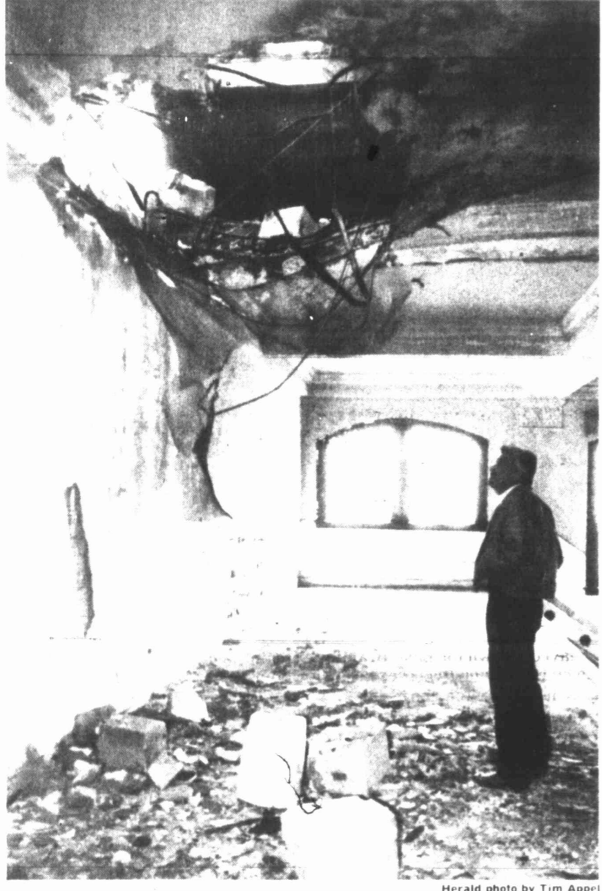
Richard Atkins looks at damage to the second floor roof of the Hotel Settles during a tour of the hotel Tuesday afternoon. Blocks on the floor were dropped from the top of the building, creating the damage.
