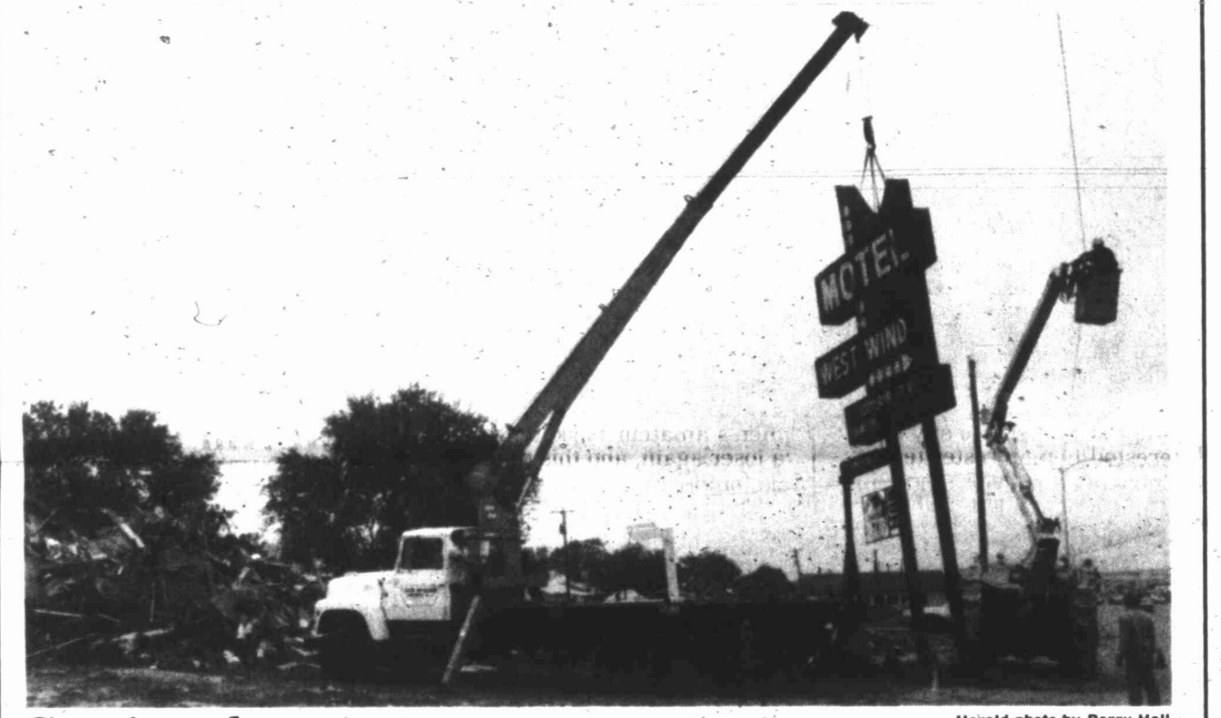
Coming down! The West Wind Motel sign, which overlooked Gregg Street for 28 years, came down to make way for a proposed H-E-B supermarket. The sign, located at 2004 Gregg, was removed by crews Thursday.
