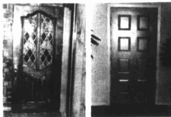
2. During this same time work begins at the home to remove existing features and in this case add an archway opening to the kitchen.
