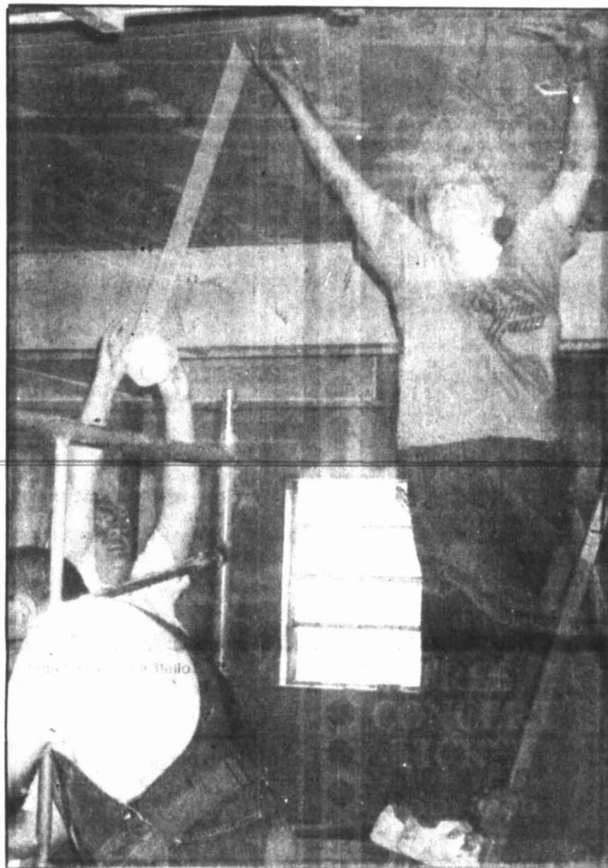
Campers on Mission volunteers Alma Simpson and Edna Ames (on the ladder) applied tape to the ceiling of the new Fellowship Hall at Baptist Temple Church this week, while Delbert Simpson, left, measured lumber for the project.
