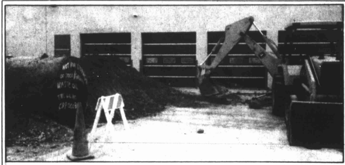
Tank removed Mt. Juliet Excavating & Construction of Old Hickory, Tenn., is removing an underground oil storage tank from the former K-Mart parking lot. The Environmental Protection Agency has ordered the removal because of possible leakage, said a company spokesman.
