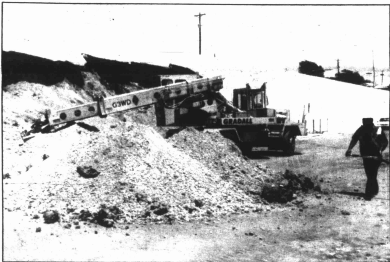
Texas Highway Department worker Robert Rodriguez assists with a shovel while maintenance crews clear dirt and cement debris from the FM-700 embankment near the Gregg Street overpass early Sunday. The weakened wall broke about 2 a.m., forcing closure of the northern-most lane for about two weeks while workers continue to monitor any movement. Securing a contract for repair may take up to two months, said Resident Engineer Mike Chetty.
