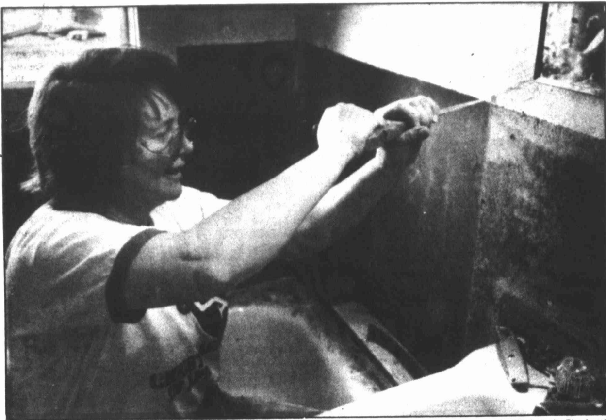
Katherine Cline uses a hand saw to smooth the edge of a piece of plasterboard that she was cutting in the bathroom of a home at 1307 East Sixth St. this morning.
