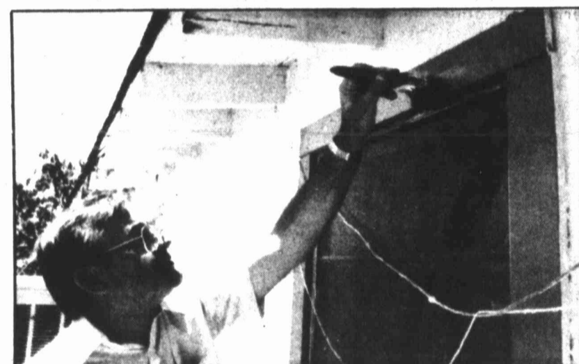
Jimmy Brunson does some touch-up work on the edging around a window at a home at 901 N.W. Third St. Saturday afternoon. Texaco employees and their families had the task of repairing the house as part of Christmas in April.
