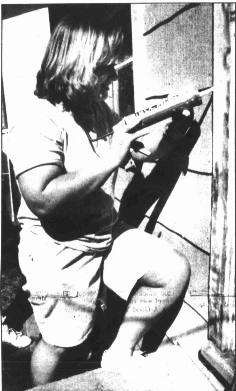
Missie McKay uses a caulking gun to apply caulk around a doorway before the house at 806 East 13th St. could be painted. Members from the Howard County Jaycees and the Church of Jesus Christ of Latter Day Saints teamed up to do major interior and exterior work.
