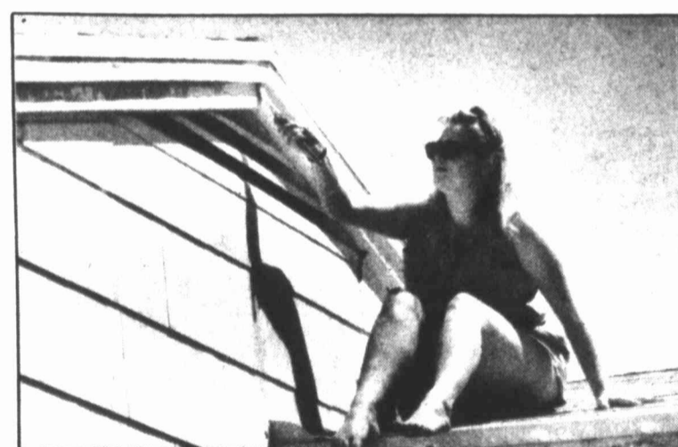
Sitting on a lower roof, Dana Kohl paints an overhang as she and others from St. Paul Lutheran Church work on a house at 1403 Stanford Avenue Saturday.
