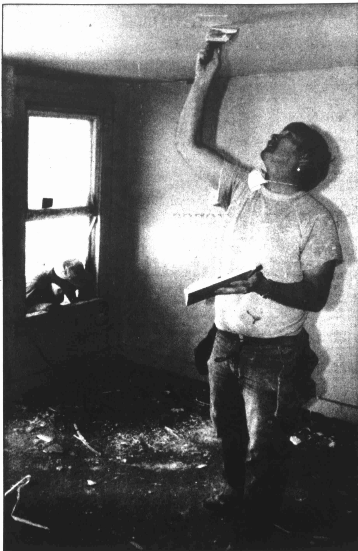
Alvin Casey reaches high to apply plaster on the living room ceiling at 602 N.E. 10th Street as he and others from College Baptist Church did roof and ceiling work, along with some cosmetic painting.
