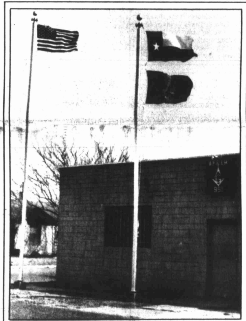
Project finished Two new flag poles were set at the Stanton Masonic Lodge No. 951 this week. According to Mason Mitch Holt, the pipe was donated by B. F. White, Donnie Thigpen donated the welding and Bob Reddon, a Grand Lodge officer, donated the Masonic flag. Lodge members donated funds to complete the project.
