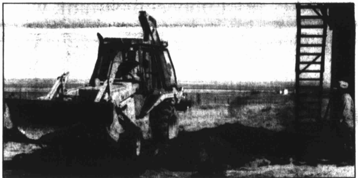
Workers take a break before completing the installation of a 500-barrel water tank between Lenorah and Stanton recently. The water tank will
