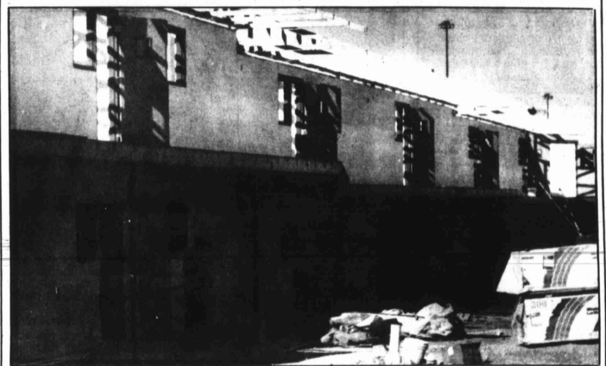
Workers, top photo, attach metal siding to the building which will house the Big Spring Correction Center II's administrative services and main entrance area. The building was originally built for Webb Air Force Base. Inmate housing
