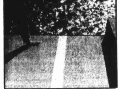
CHECKING DAMAGED BRIDGE
