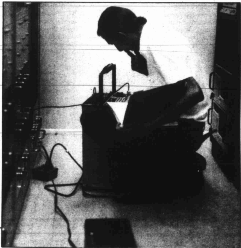
Bruce Carby, an employee of Westex Telecommunications of Stanton, works to align radio equipment at Westex's cell tower station south of Big Spring. The communications company is expected to start providing cellular telephone service to this area sometime next month.
