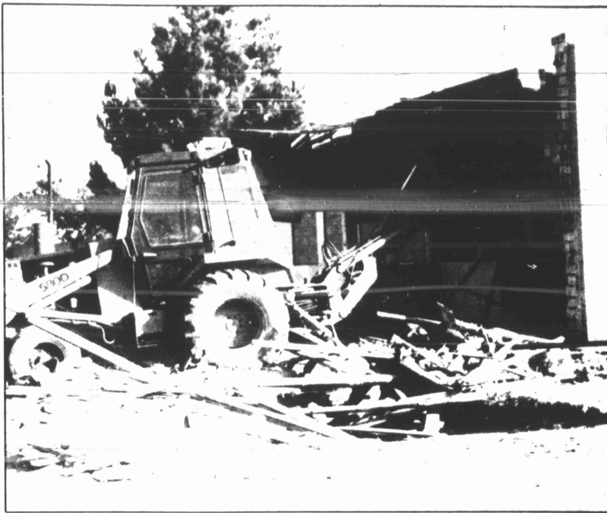
STANTON — Walls of the old Cap Rock Refrigeration Cooperative are coming down as the building is razed.
