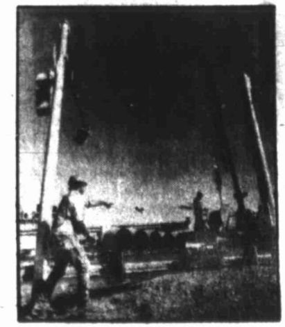
BIG SPRING — City employees put up new traffic lights in Big Spring recently.
